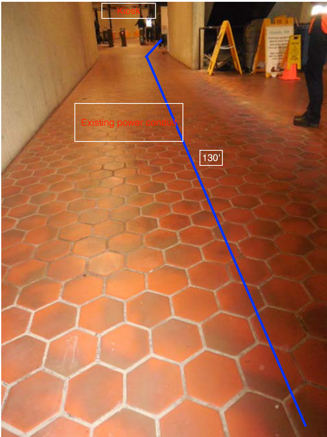
Photo #1 – Existing power conduit on mezzanine floor.
