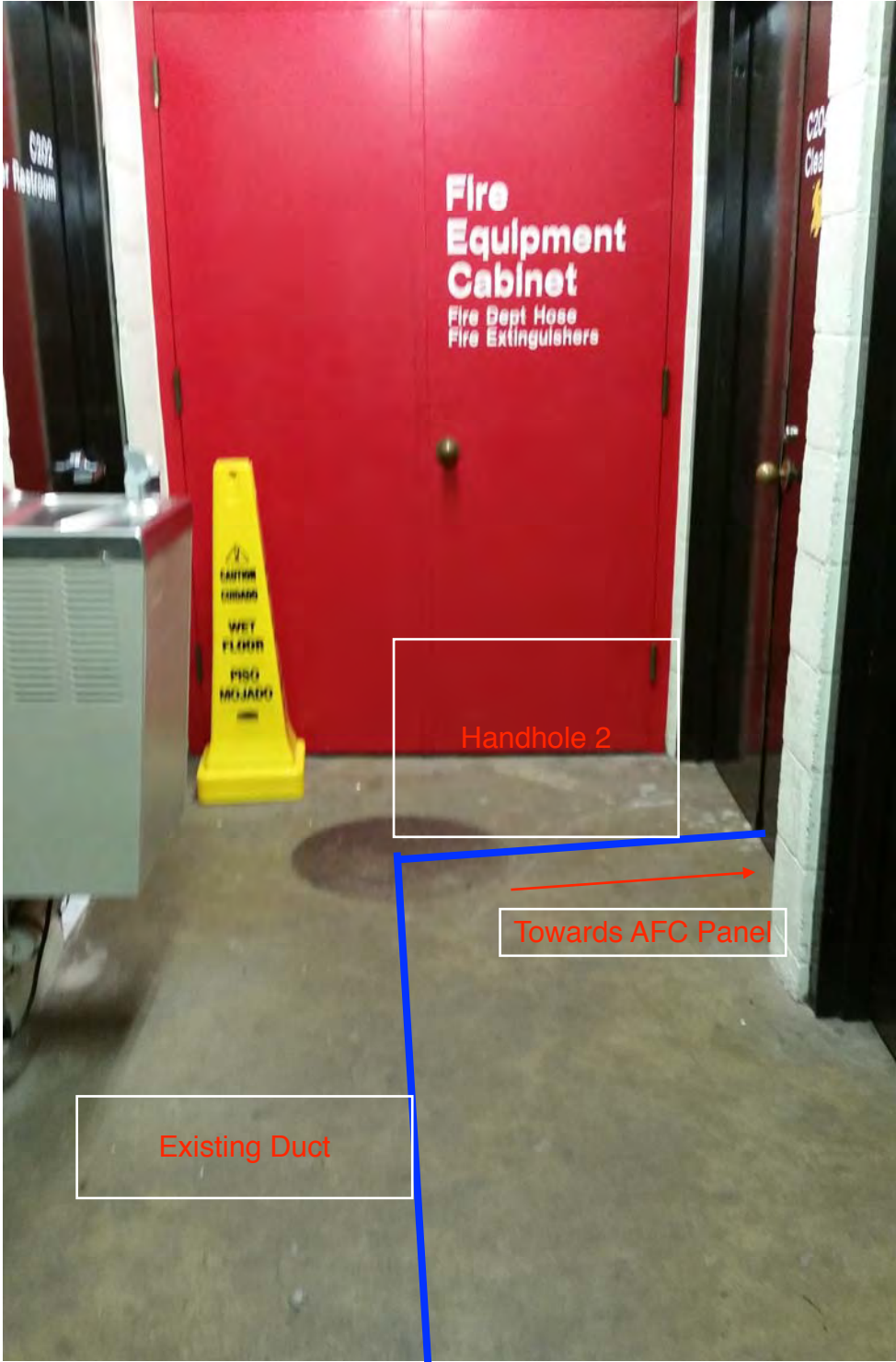
Photo 3 – Handhole 2 in Room C200.
